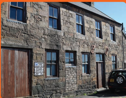
South Pier House , attached to La Folie Inn, owned by Ports of Jersey. Adapted in 1926 from older buildings to form a house; listed building Grade 4. Vacant, Boarded up for years and awaiting redevelopment.
